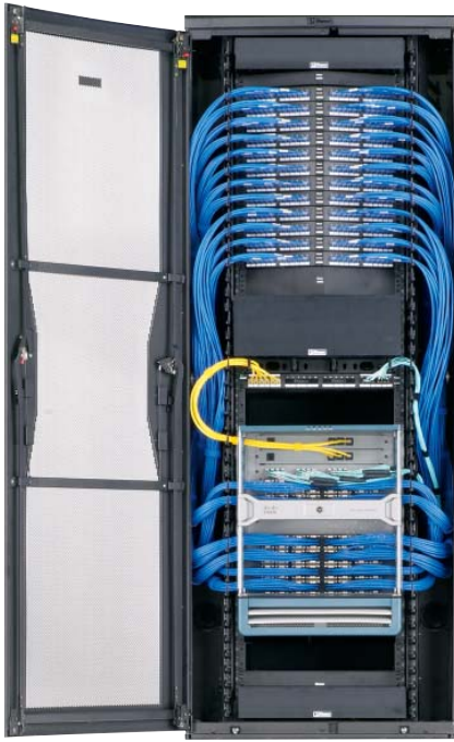
(Nexus 7009 "Heavy Copper" Pre-Configured Physical Infrastructure shown)
